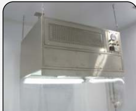
Ceiling Suspended Laminar Air Flow
